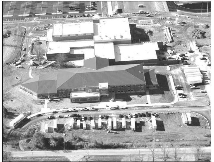
Above is an aerial view of the high school construction site on April 11, 2011.
